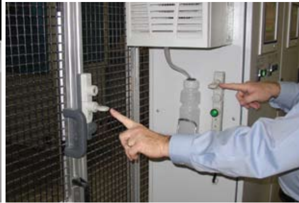
Here is a view of the safety fence with a double-key lock to secure the shuttle area where goods emerge from the tunnel. Unauthorized entry will cause the entire system to shut down.
