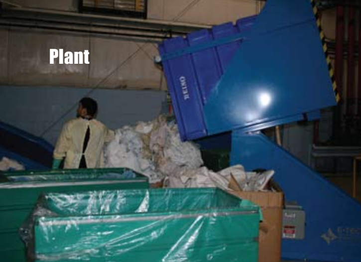
A cart dumper deposits soiled linens near a ramp where they'll soon move up to the sorting area. Bulk items such as sheets that don't require sorting will go onto a center belt that moves them to a sling that goes directly to the tunnel washer.
